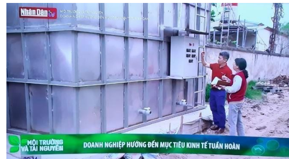
WWTP for circulation in the Vieba Garment Co. Ltd. (Nhandan TV Channel)
